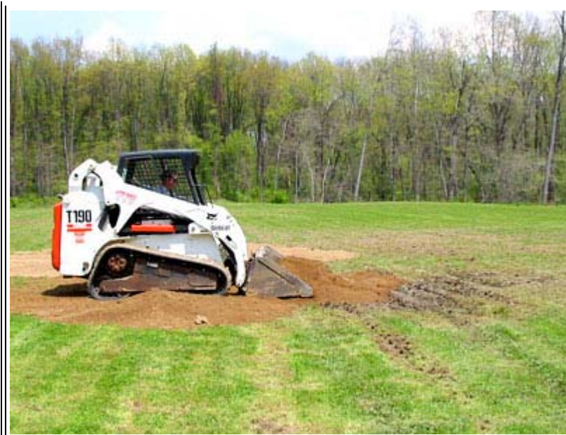
An uneven grading job resulted in low spots that collected water and created hazardous, muddy conditions. Here the skid steer operator moves topsoil to fill the low spot.
